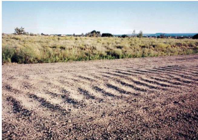
A typically washboarded road
